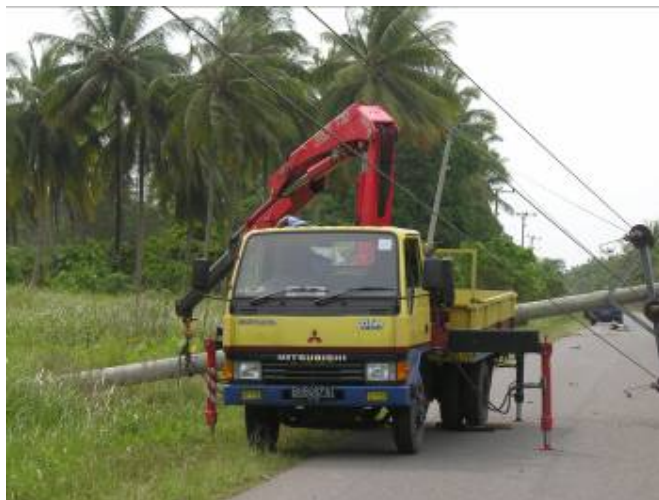
Electricity facilities are still under repair by local government
