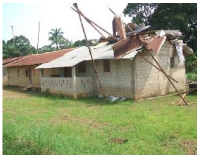
Wind-damaged house in Gabon , January 2011 /photo GRCS
