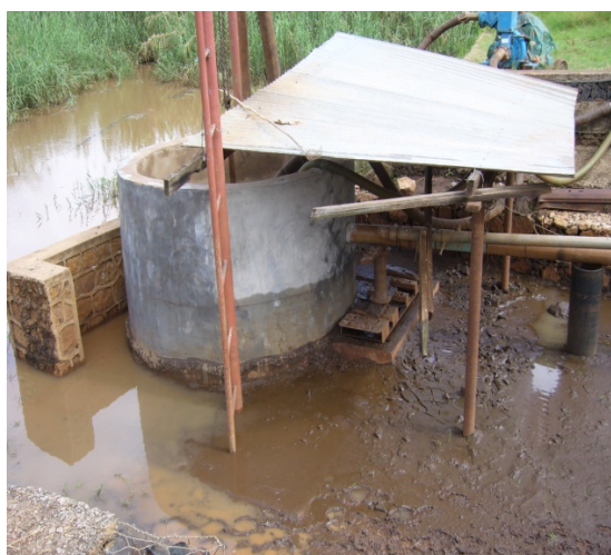
The water source at Mkandage in Kilosa
