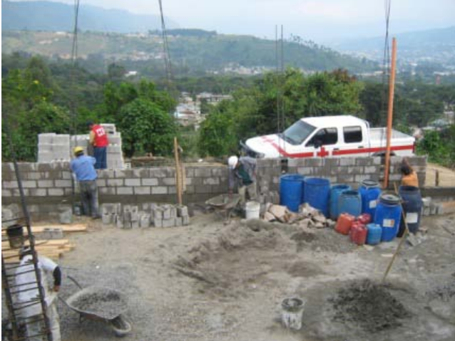
The Guatemalan Red Cross has initiated its shelter programme, building and maintaining collective centres, as well as providing construction materials to affected families. Photo: Guatemalan Red Cross.
