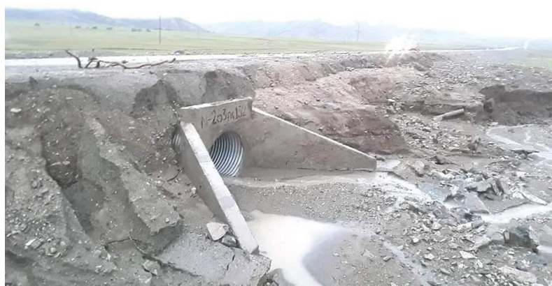
Bulgan to Khuvsgul province road is damaged. (Photo: Ikon.mn)
