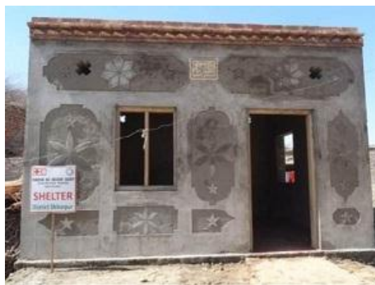
A completed shelter beautifully plastered by a beneficiary in Sindh province. Photo: IFRC.
