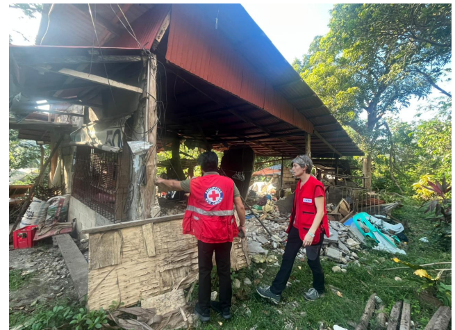
Joint shelter damage assessment by the PRC and IFRC in the municipality of Tabuelan in Cebu province. (Photo: IFRC)
