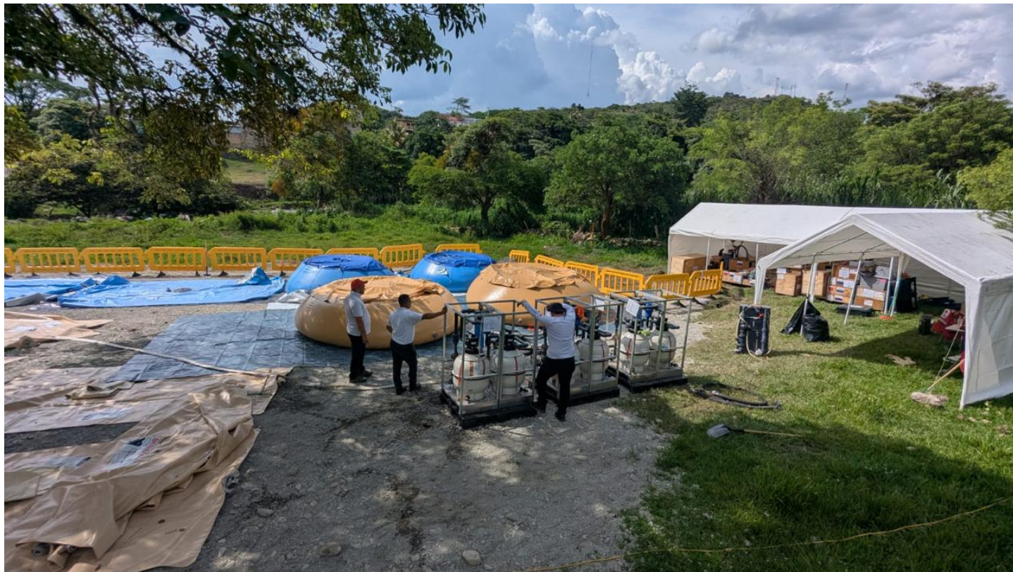
M15 plant: water treatment & distribution, July 2025, Ocotepeque.
