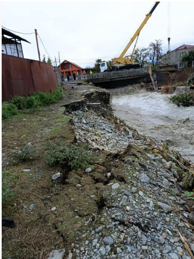
Damaged riverbank. Photo: Georgia Red Cross Society (GRCS)
