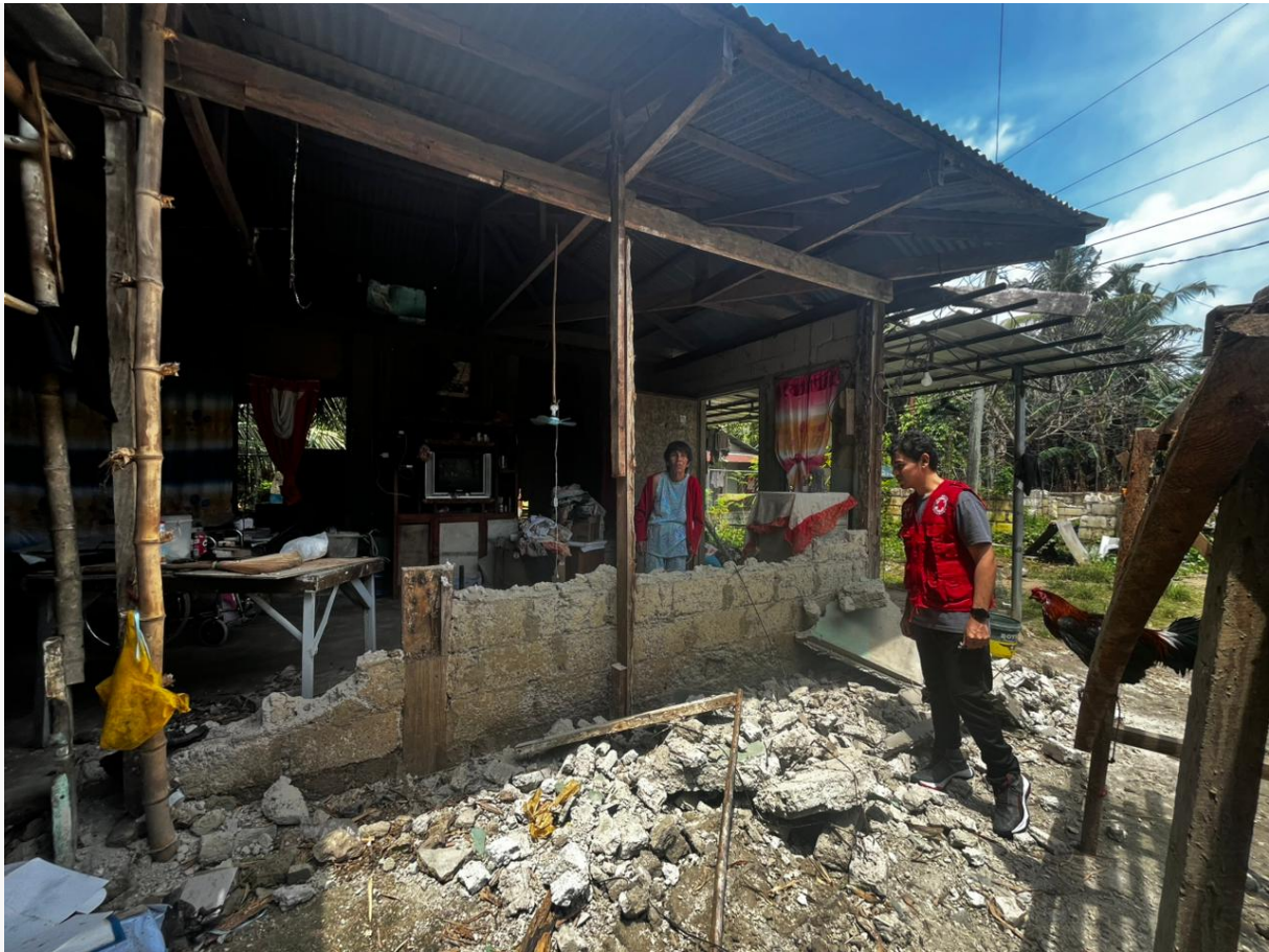
Reduced to rubble-the quake stole more than walls, it stole lives. (Photo: PRC)
