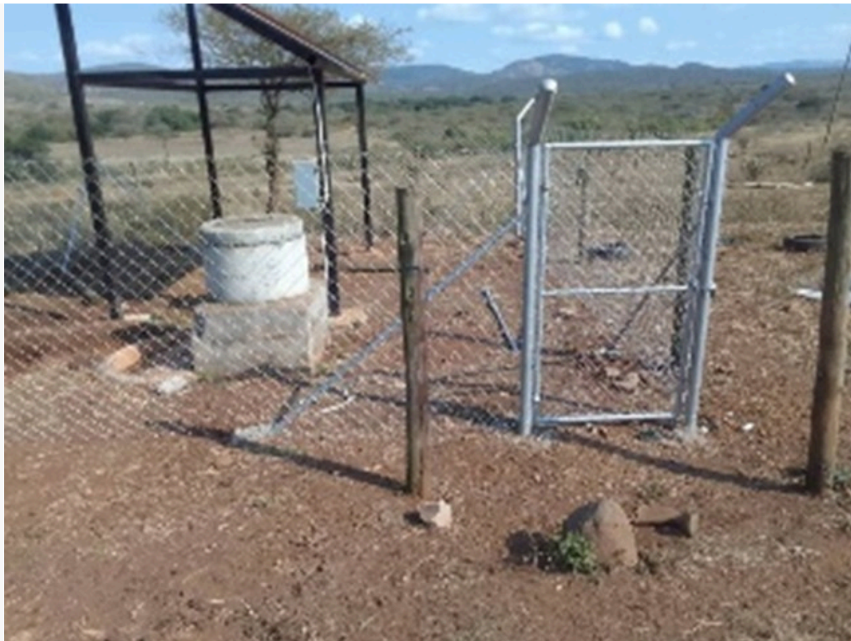
Fenced water point supported by the project at Stilo, Matsanjeni
