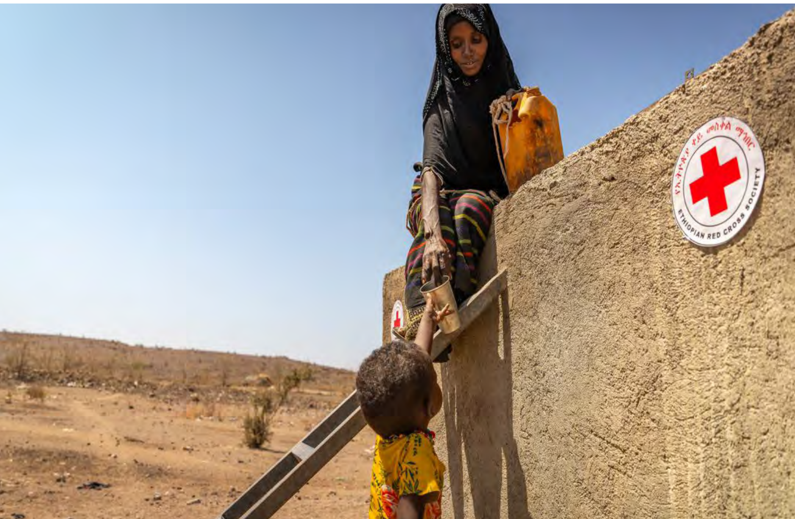
The construction of smaller storage for safe drinking water provides support to families to gather and store rainwater. (Photo: Finnish Red Cross)
