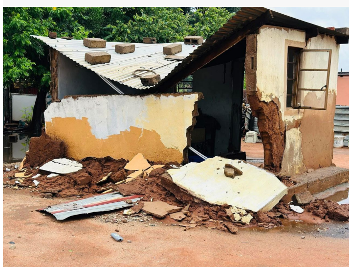
House collapse following floods in Tlokweng
