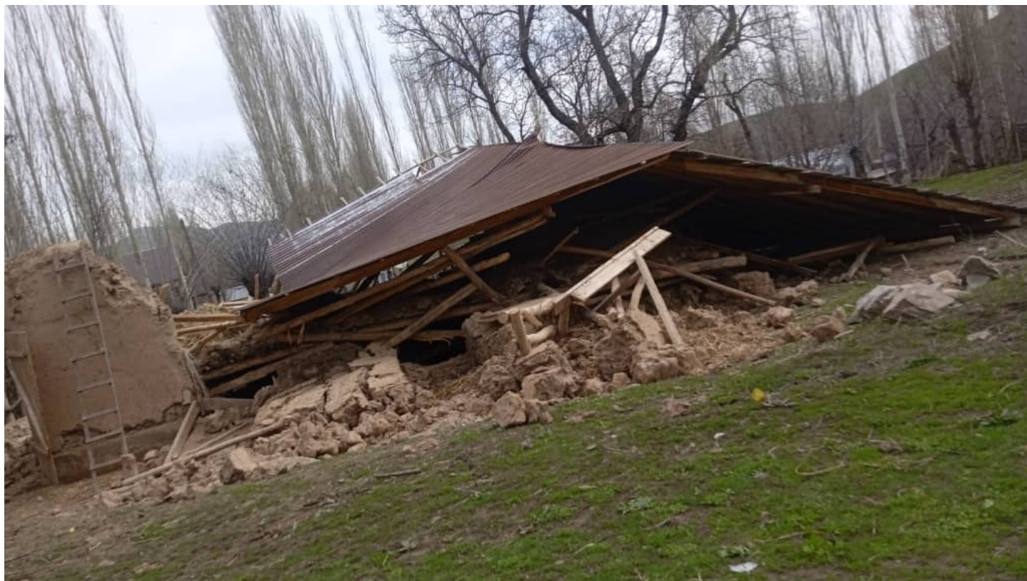
Fully destroyed house in Rasht. Photo credit: Red Crescent Society of Tajikistan
