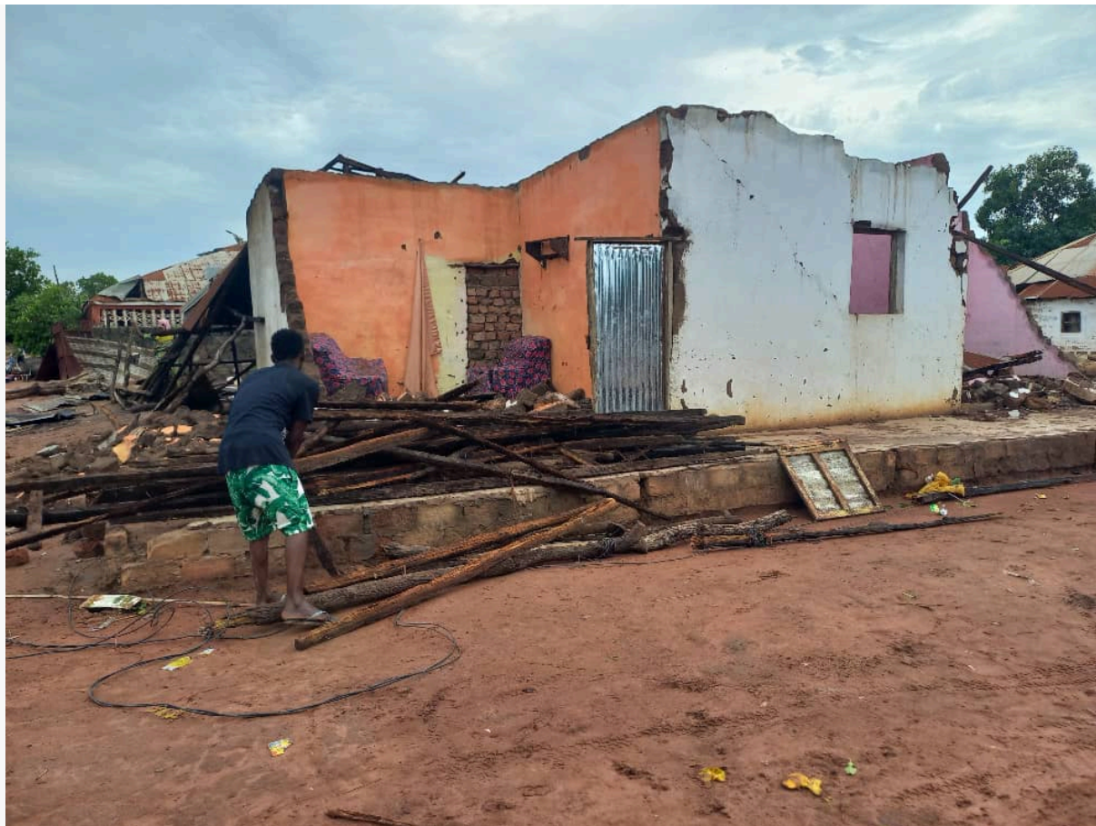
A completely damaged house in Gabu community
