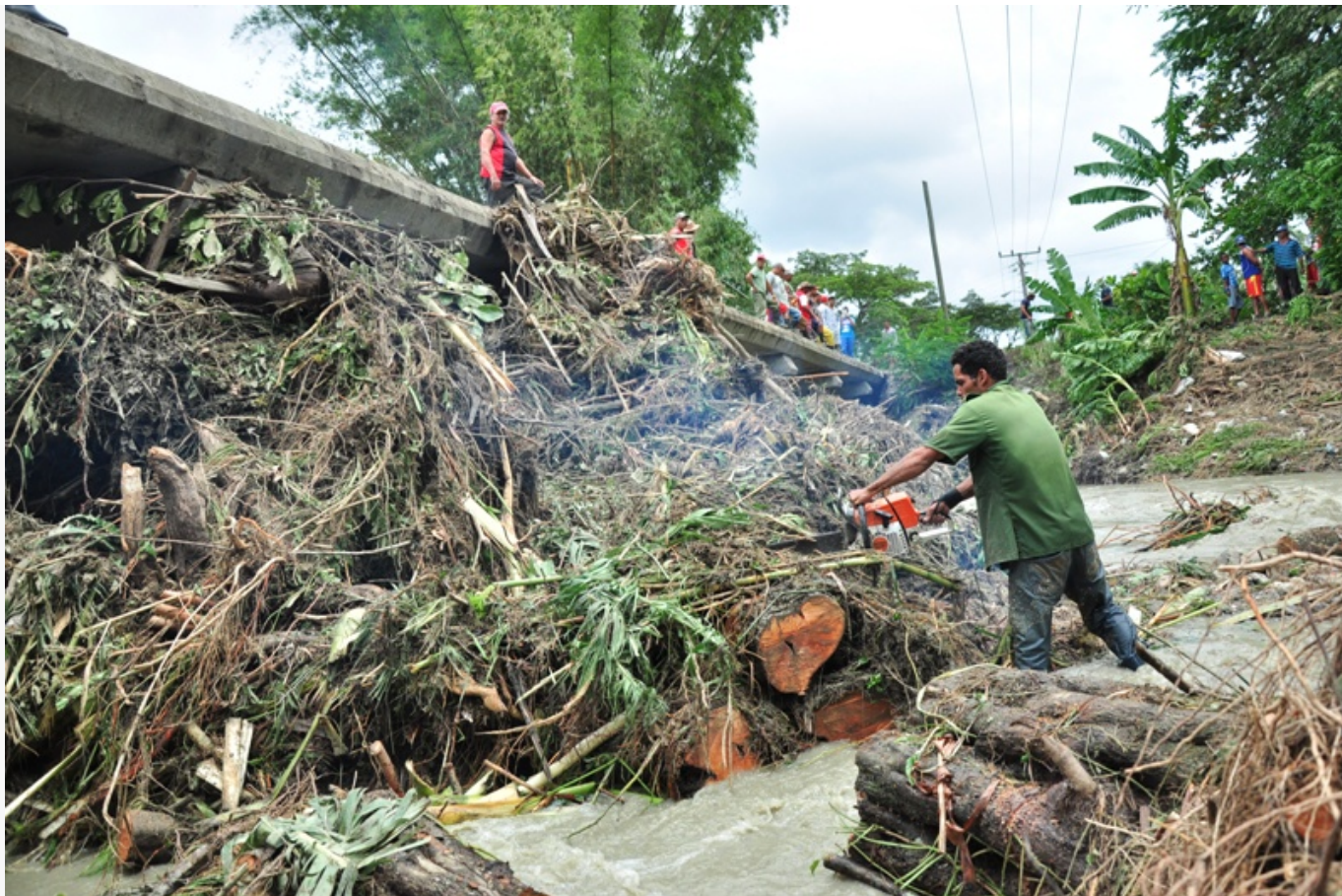
Debris removal on roads in San Antonio del Sur, Oct 2024. Source: CRC
