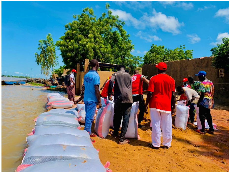
Photo 1: Placing sandbags in the commune of Sofara, to prevent houses from getting flooded
