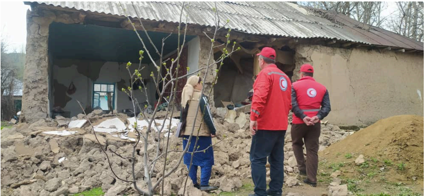
Damage assessment by RCST team. Photo credit: RCST.
