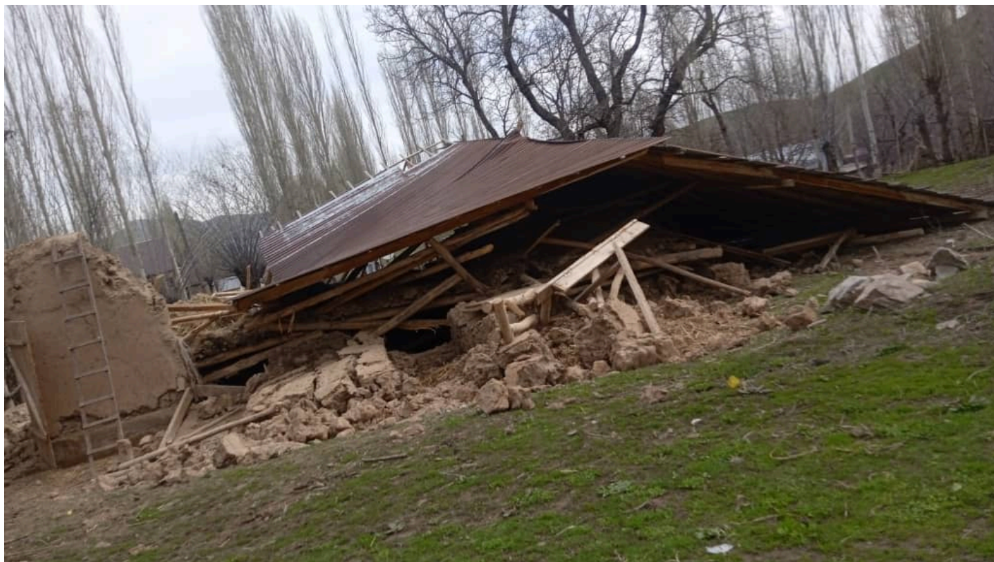
Fully destroyed house in Rasht valley. Photo credit: The Red Crescent Society of Tajikistan (RCST).
