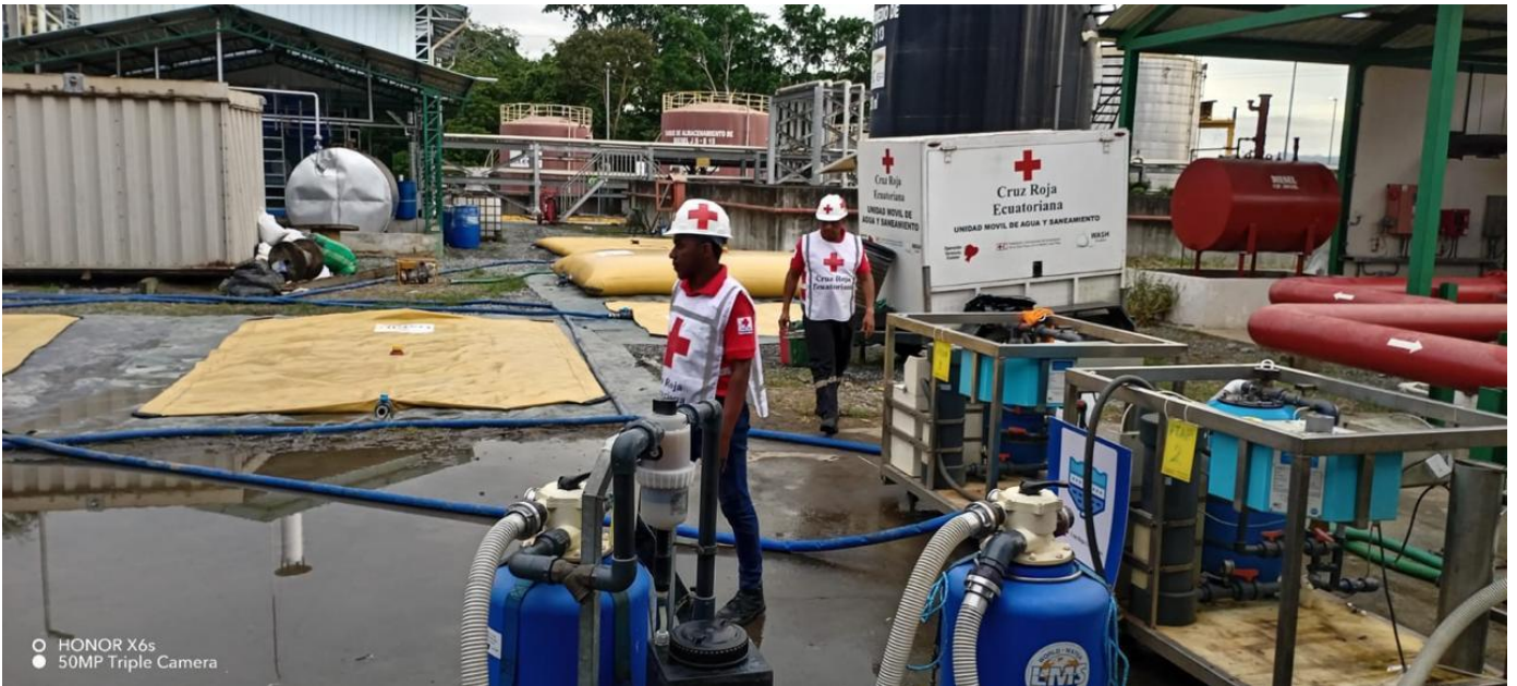
On 20 March 2025, Ecuadorian Red Cross teams installed a N.5 kit to produce drinking water at the Esmeraldas thermoelectric plant.
