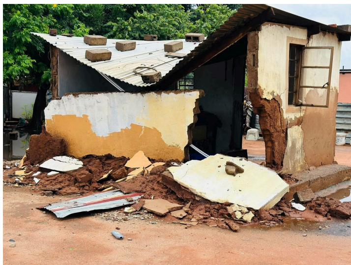
House collapse following floods in Tlokweng
