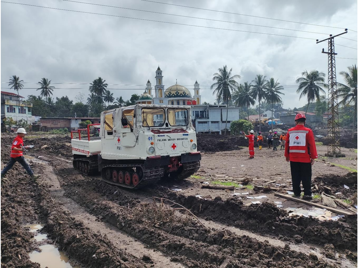
Post-flood cleanup in Agam, West Sumatra Province, carried out by PMI personnel alongside the local community and government. (Photo: PMI)
