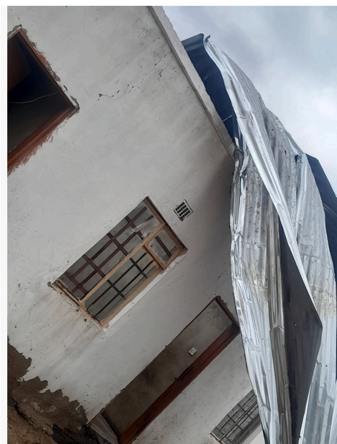
Damage in Mogoditshane
