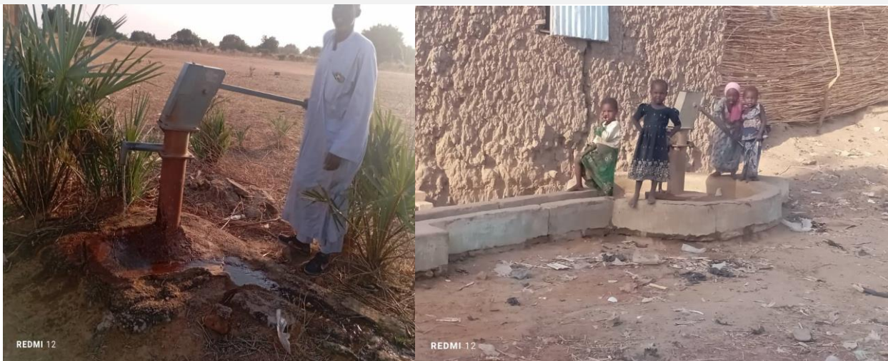
Some water points rehabilitated by the Chad Red Cross in Massenya in the Province of Chari Baguirmi
