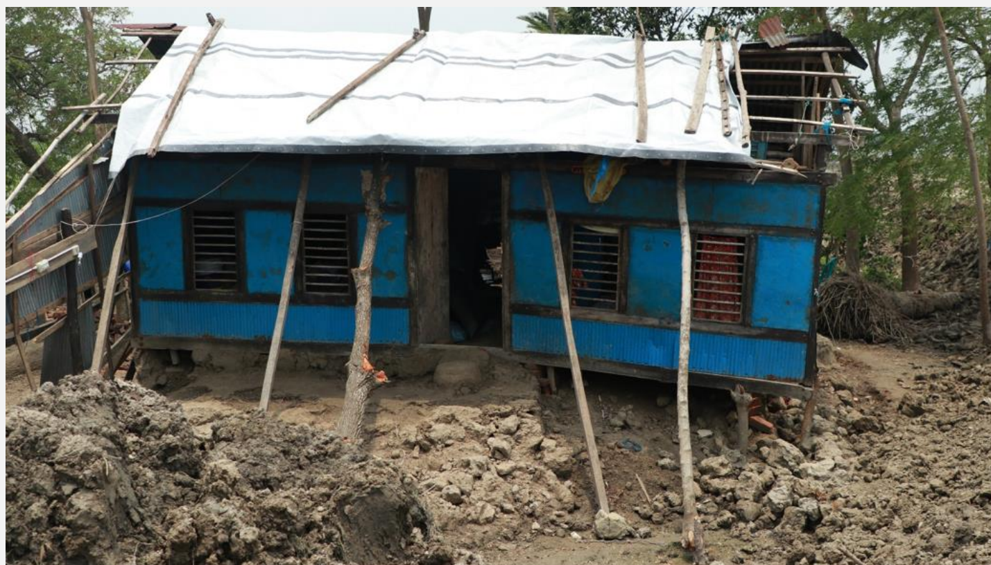
One of the damaged houses temporarily uses tarpaulin as a rooftop in Morelganj, Bagerhat, following Cyclone Remal (Photo: IFRC)
