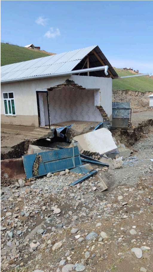
Mudflows severely damaged and destroyed houses. Photo: RCSK.
