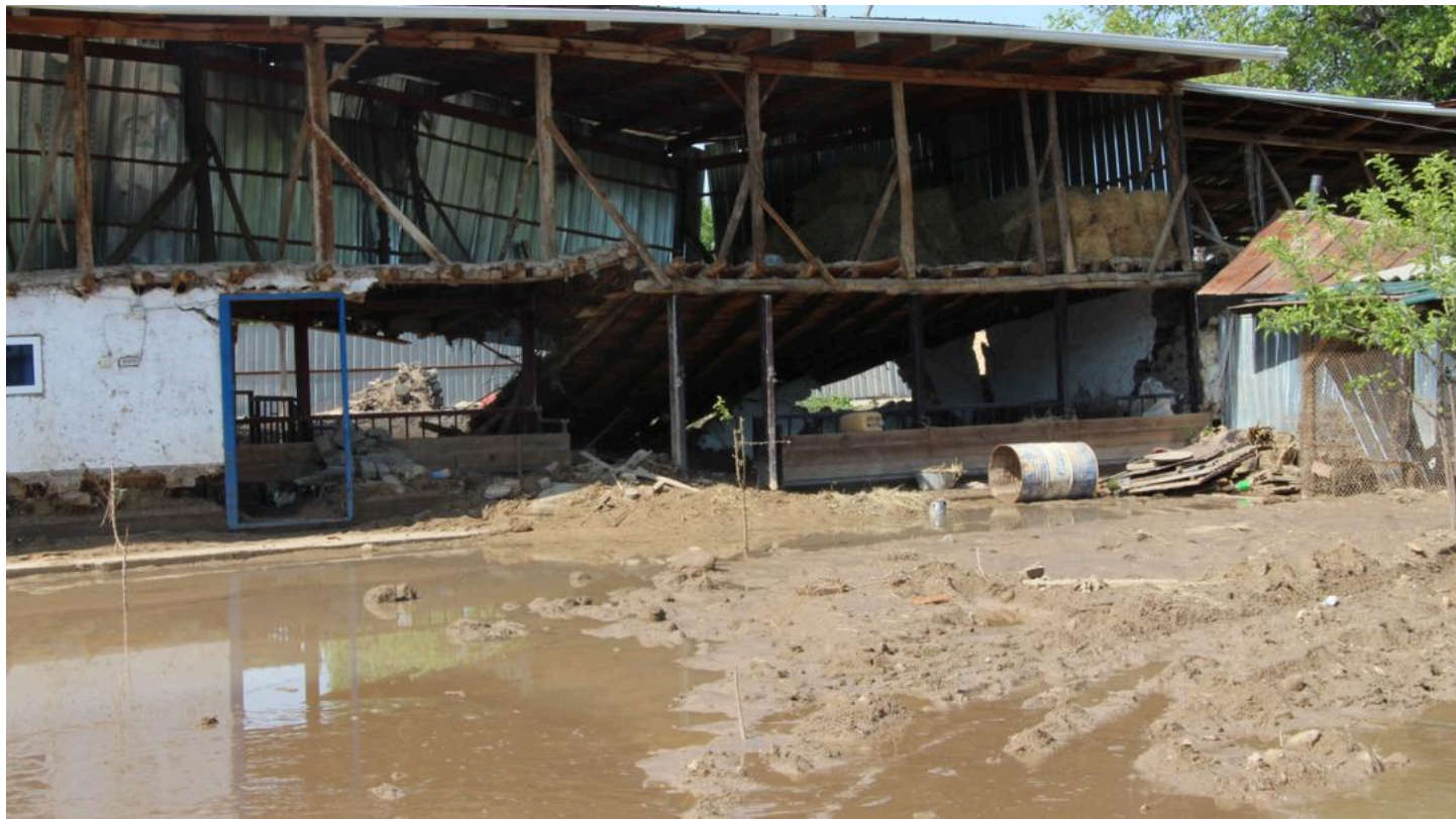
April floods caused extensive damage. Photo: Red Crescent Society of Kyrgyzstan.
