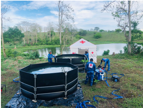
Operation of water purification plant in the department of Cordoba, May 2024. Source: Colombian Red Cross
