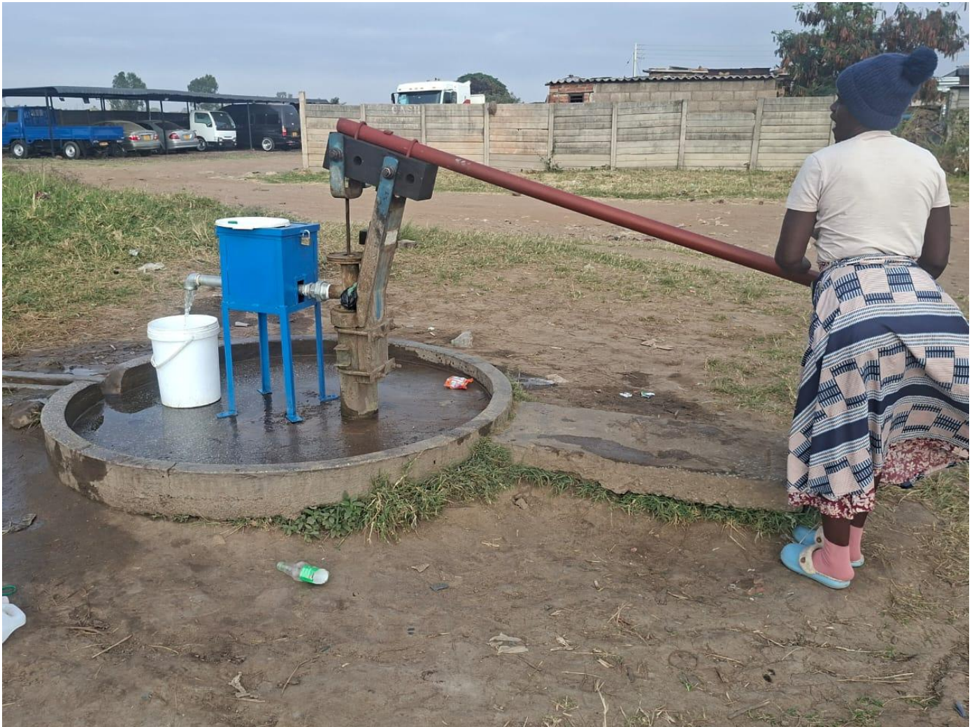
Figure 1: Newly installed inline chlorinator in Glen-View, Harare, Zimbabwe, Photographer: Dorika Madzingamiri, DFO, ZRCS
