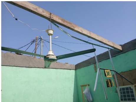
Houses damaged by windstorm in Dhikil; Djibouti, Photo Credit_ DJRC Volunteers
