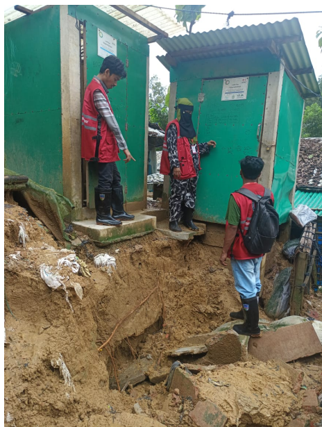
Heavy rainfall caused severe damage to latrines (Photo: BDRCS)
