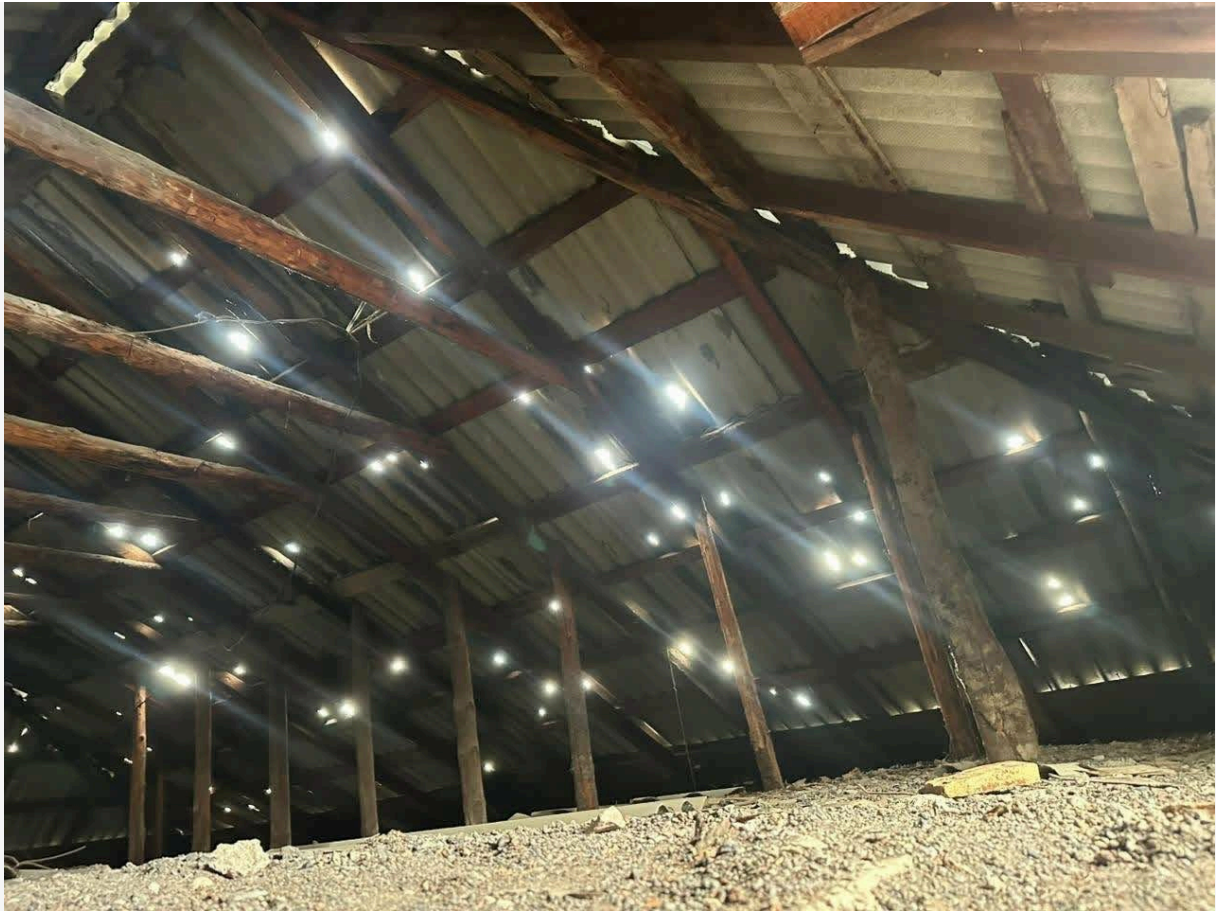
Severe hail damage to residential roofs, Stepanavan. Photo credit: ARCS
