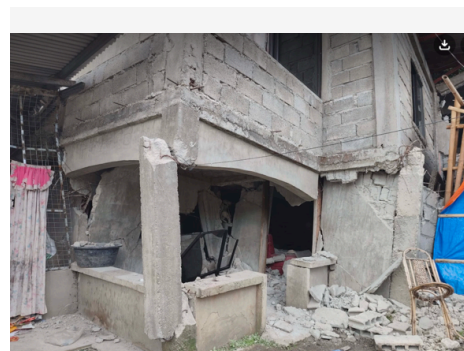
A residential home severely damaged by the earthquake in, South Cotabato
