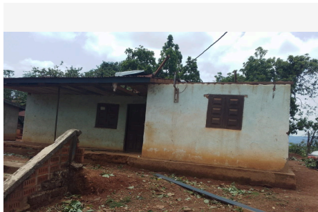
Affected house by the windstorm in Falaba District
