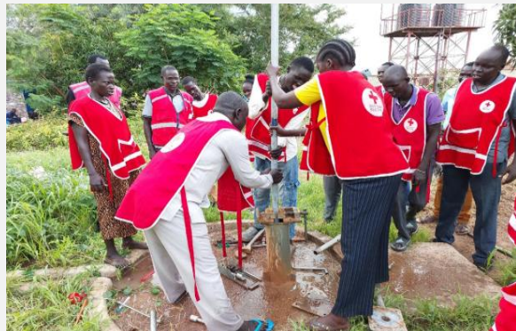
Pump mechanic participants practicing repair of borehole on 24th of July 2025 in Kuajok branch borehole,
