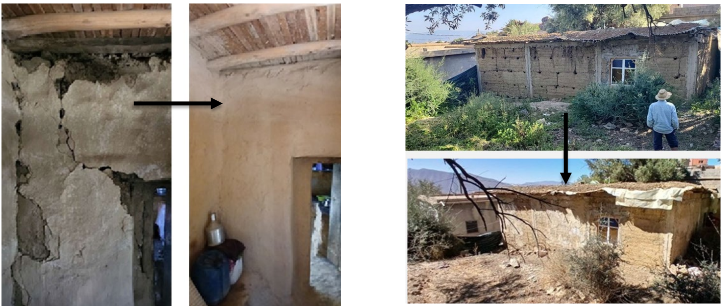
Photos 3 – Before-After photos for houses were repaired under the Community-Driven Shelter Repairs initiative. Photos: MRCS
