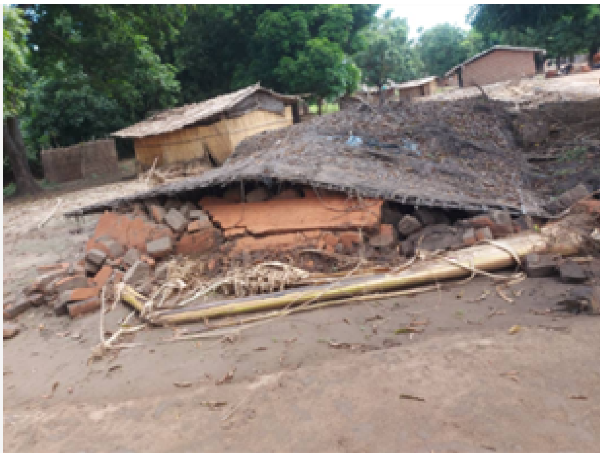
Some damaged households in Mchinji District @MRCS
