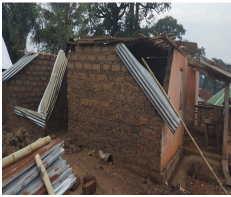
windstorm destroyed Nimba County
