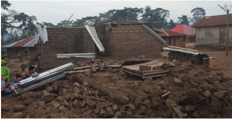
DESTROYED HOUSES NIMBA COUNTY
