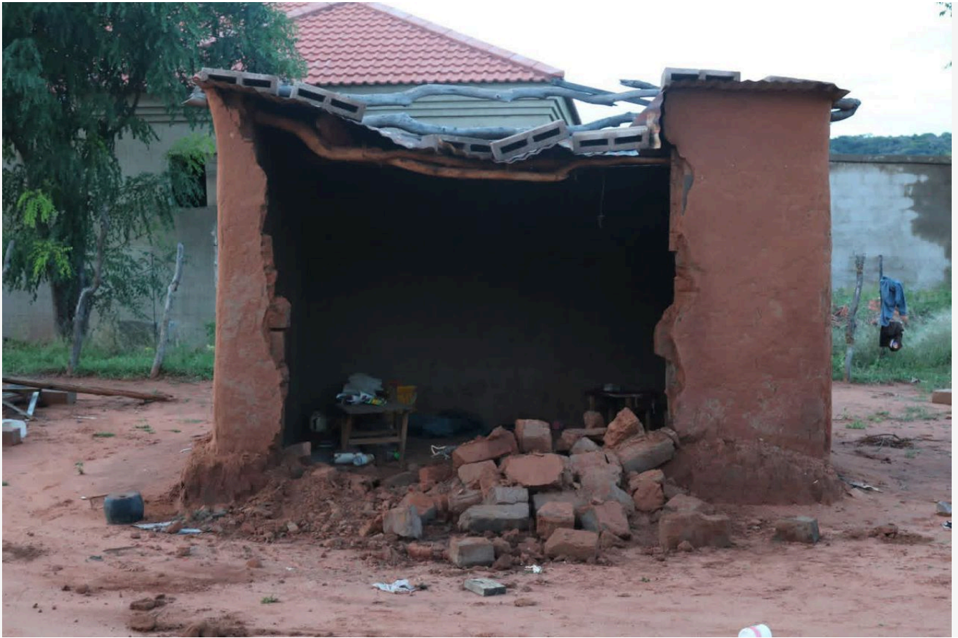
Extent of household damage following heavy rains in Lerala. Source :BRCS Comms
