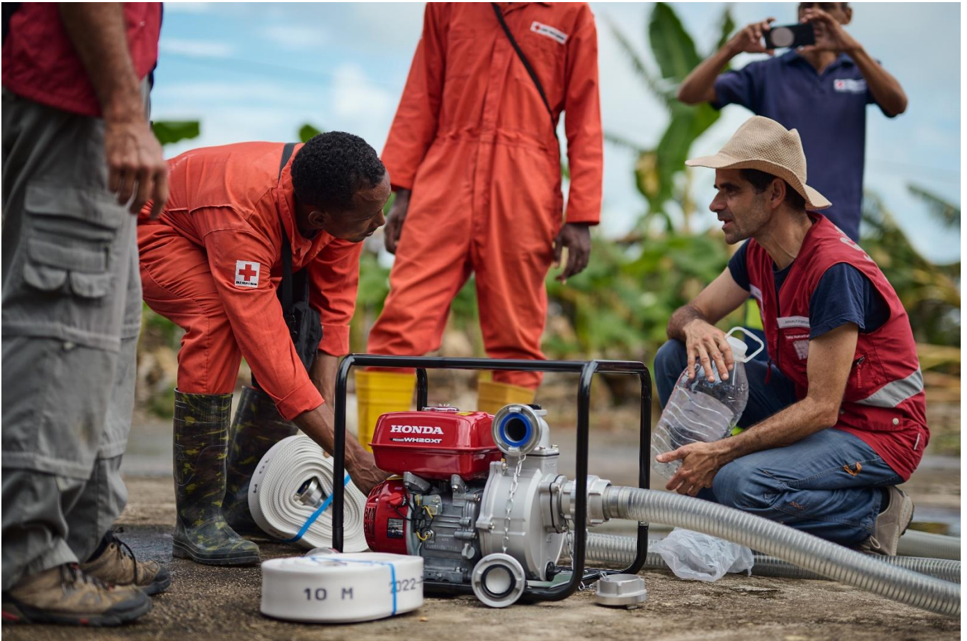
The Cuban Red Cross team is preparing the installation of a water purification plant at the San Luis hospital in Santiago de Cuba, where the drinking water supply was interrupted after Hurricane Melissa.
