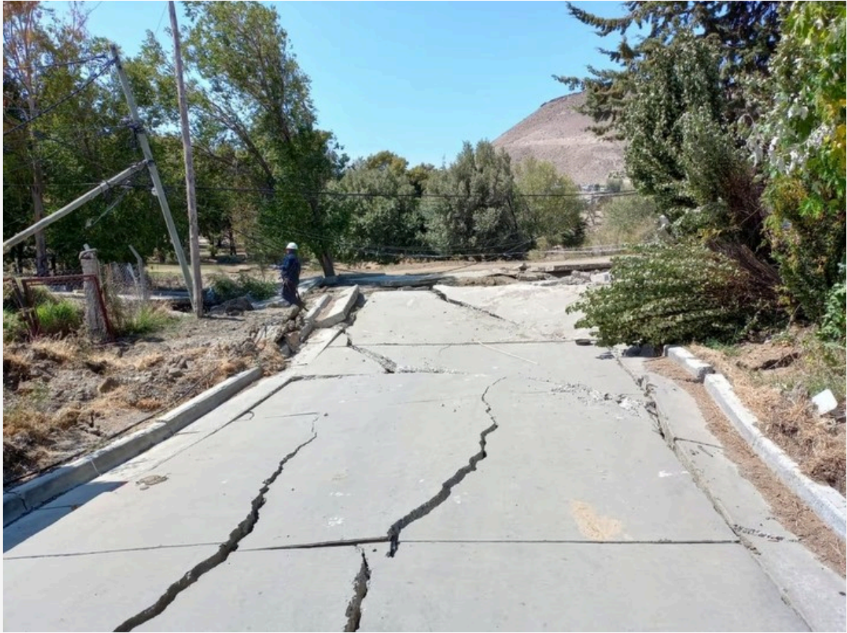
Landslide at Cerro Hermitte prompted the evacuation of hundreds of families.
