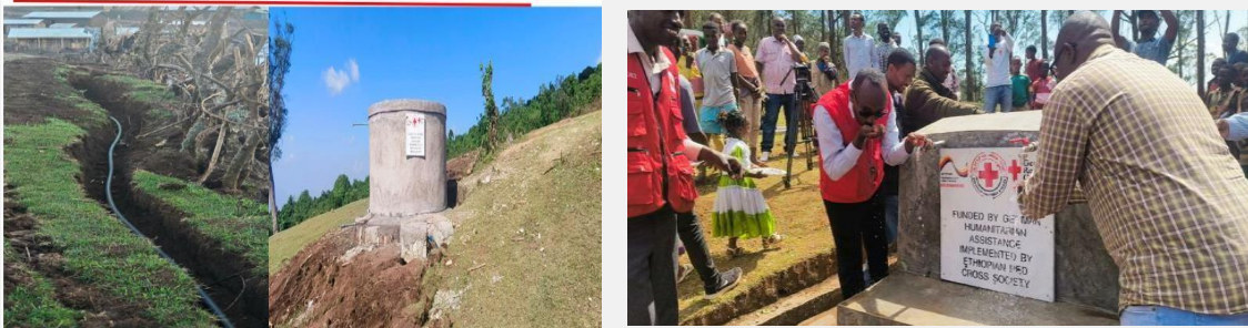
Figure 9: Water tank construction and line extension to a collection point (Bono) in new settlements in Gofa by the GRC support; photo credits ERCS Zonal Branch
