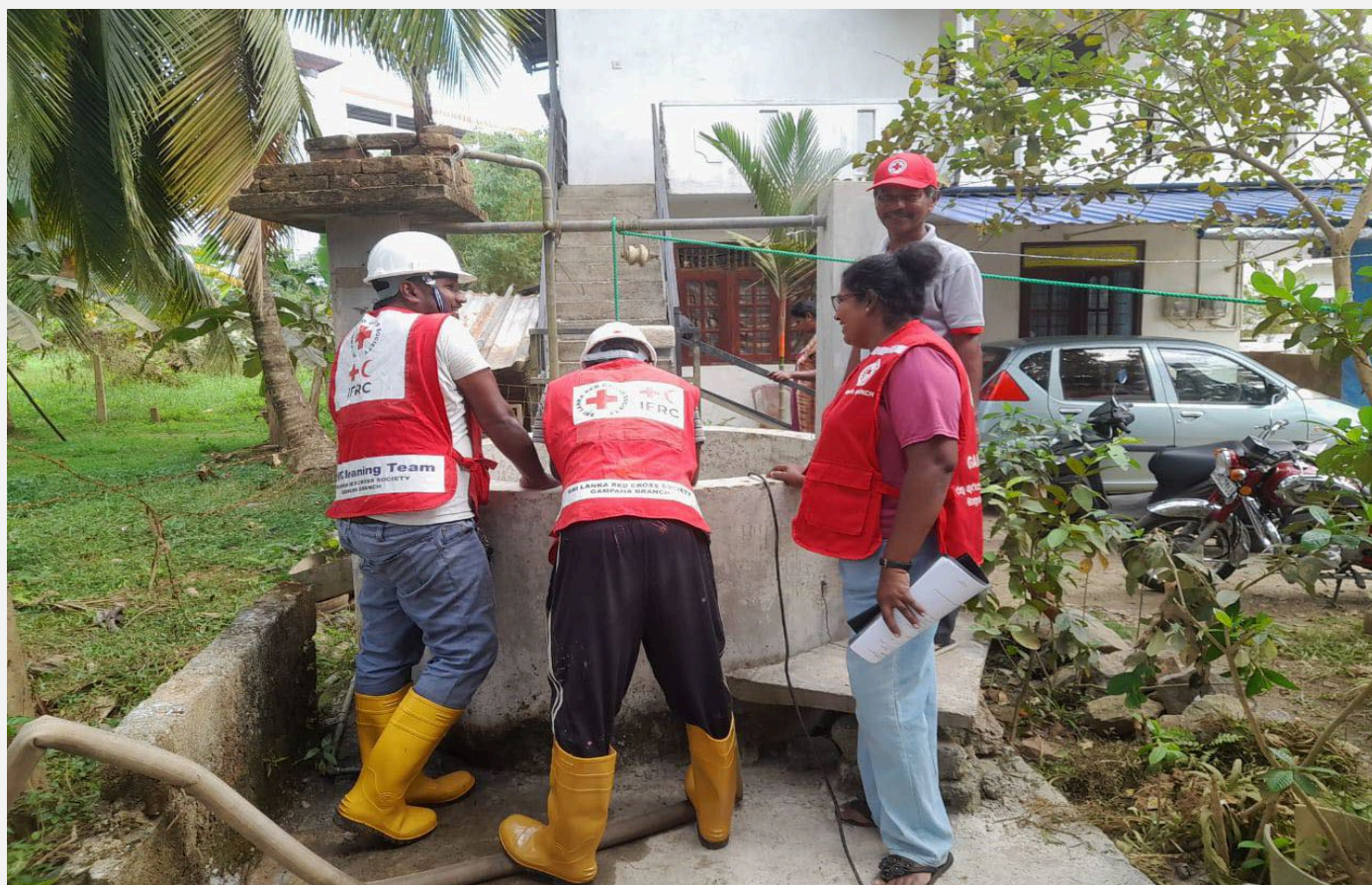
SLRCS teams carry out well-cleaning activities in affected areas, helping communities regain access to safe water. (Photo: SLRCS)
