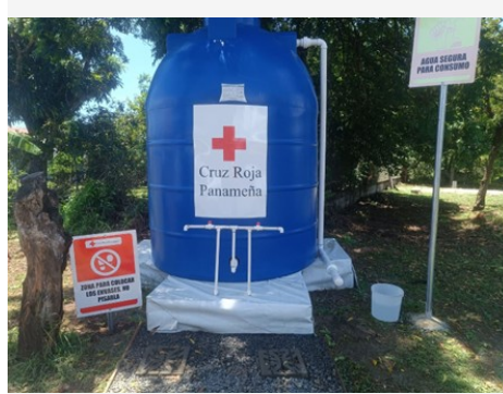
RCSP water reservoir, La Villa, Los Santos, October 2025. RCSP
