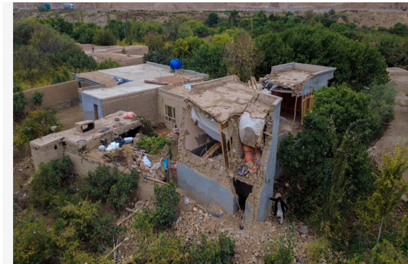
The house affected by the earthquake in Balkh Province. (Photo: ARCS)
