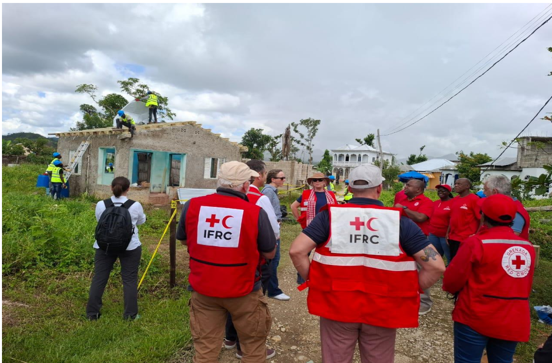
First roof repairs implemented in April by Red Cross-trained carpenters as part of recovery efforts in St. Elizabeth Parish.
