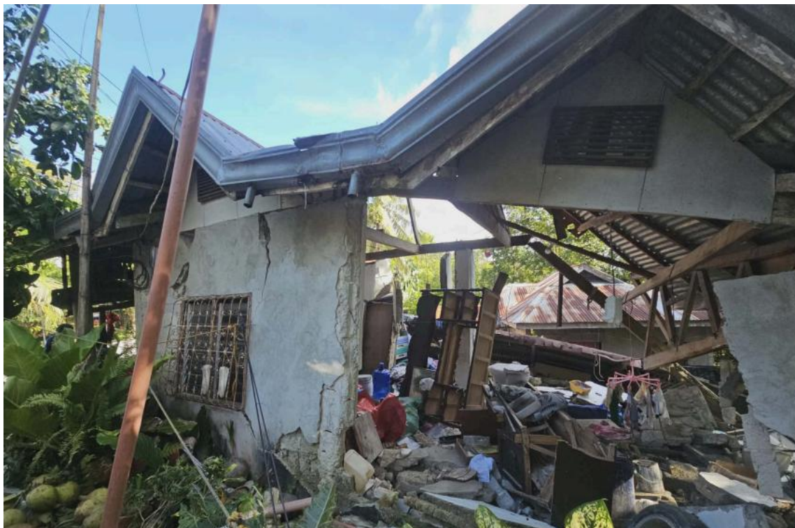
Totally damaged house in Barangay Guadalupe, Bogo Cebu City. (Photo: PRC)
