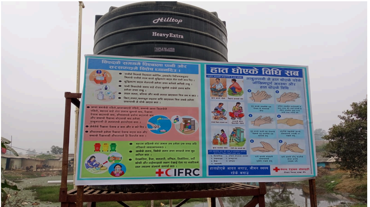
New water tank installed with hygiene messages in impacted districts.
