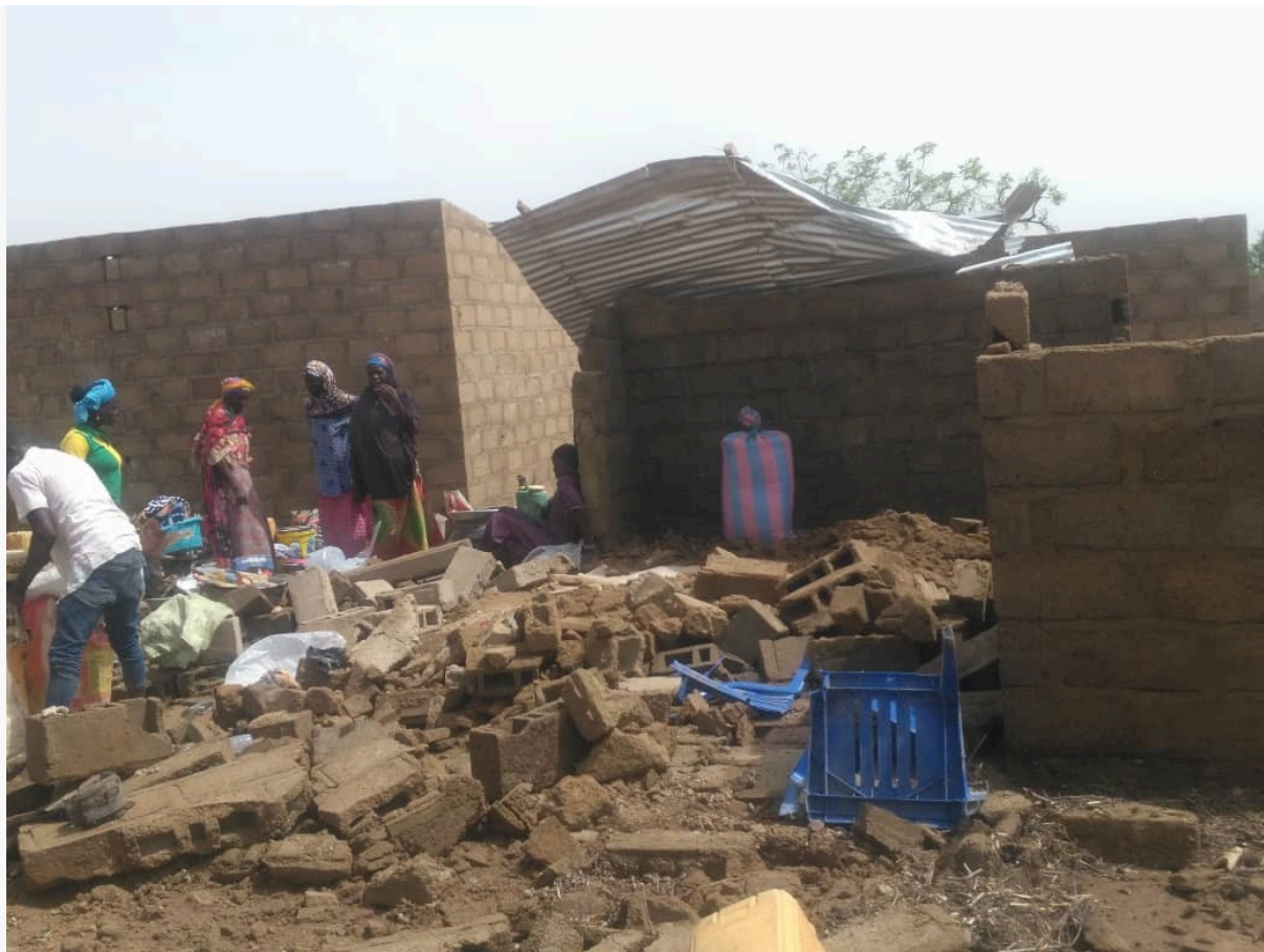
Collapsed houses in Boulsa
