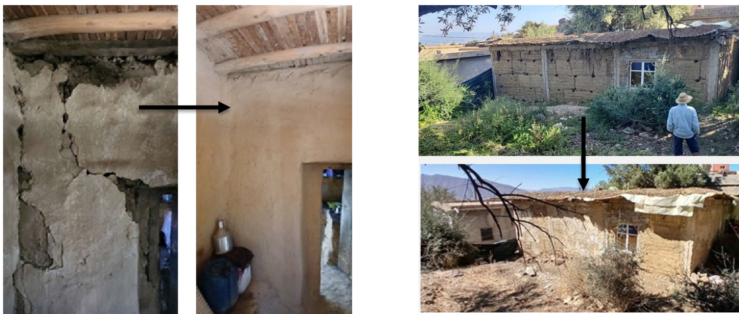
Photo 3 – Before-After photos for houses were repaired under the Community-Driven Shelter Repairs initiative
