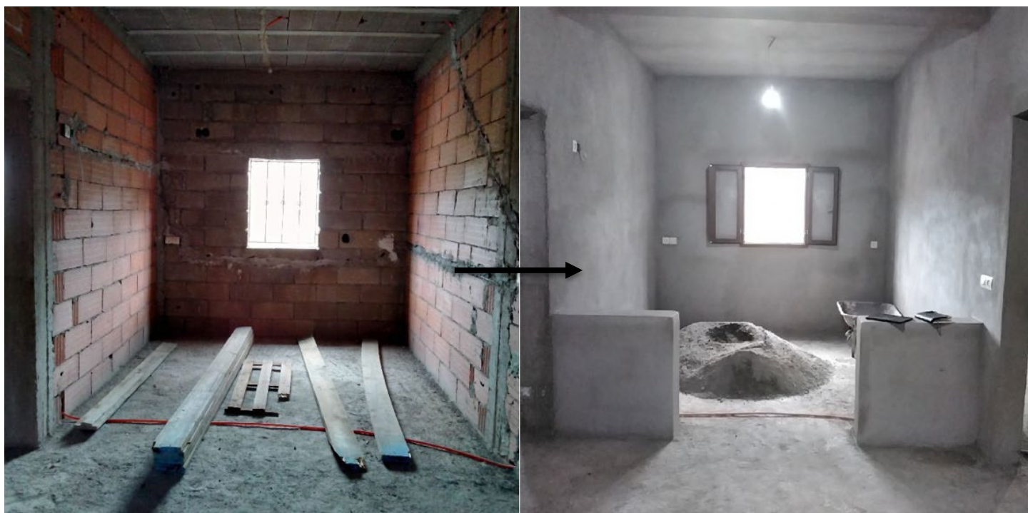
Photos – Before and after photos of a house in Taroudant Province where a family completed finishing works using top-up cash assistance under the Rapid Cash for Shelter Programme by MRCS/IFRC, complementing government reconstruction support.
