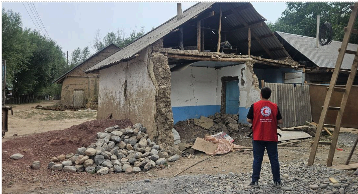
Photo credit RCST: Partially destroyed house, Ghanishob, Tojikobod
